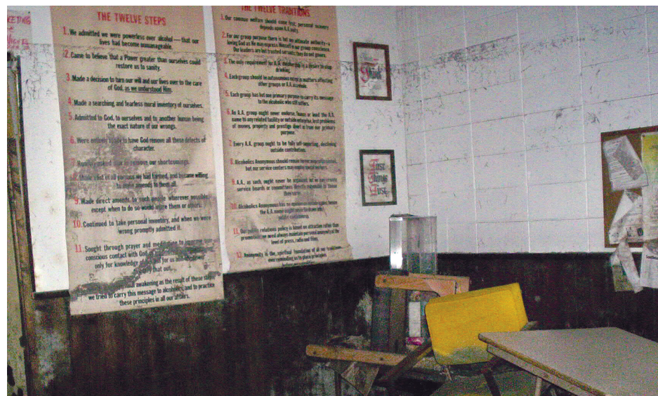
This meeting space in Chalmette, Louisiana, which was home to A.A. groups like "Ladies Night" and "Arabi We Share," shows the effects of the surging waters that inundated the area in the wake of Hurricane Katrina. Visible high up on the wall and the Twelve & Twelve shades—just under Step One—is a water stain line indicating the reach of the flood.
